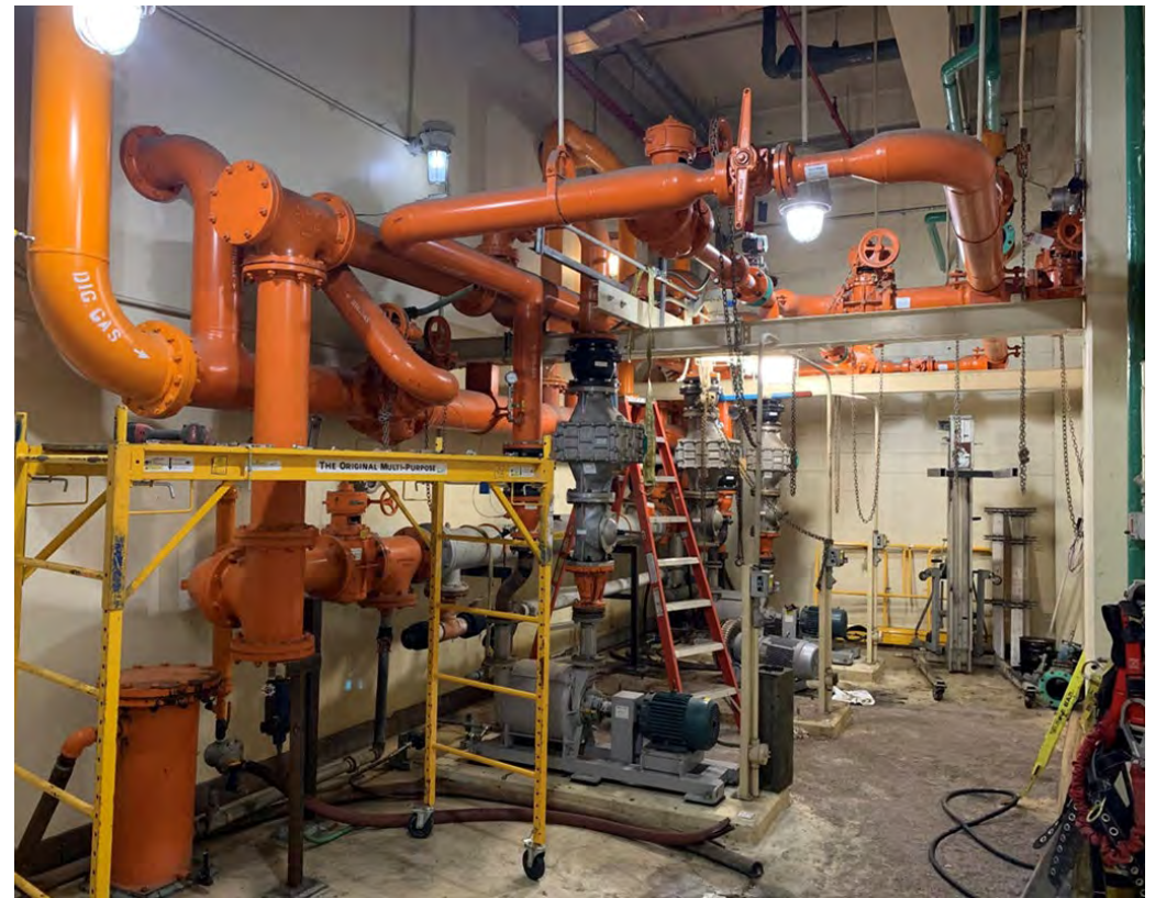
Digester Gas Blower Room (delivers digester gas to boilers).
