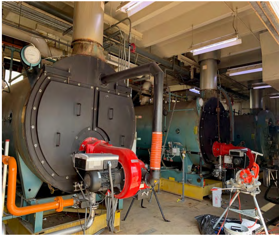
Boiler modification required to run on natural gas (NG), Blended gas (BG), or Digester gas (DG)
