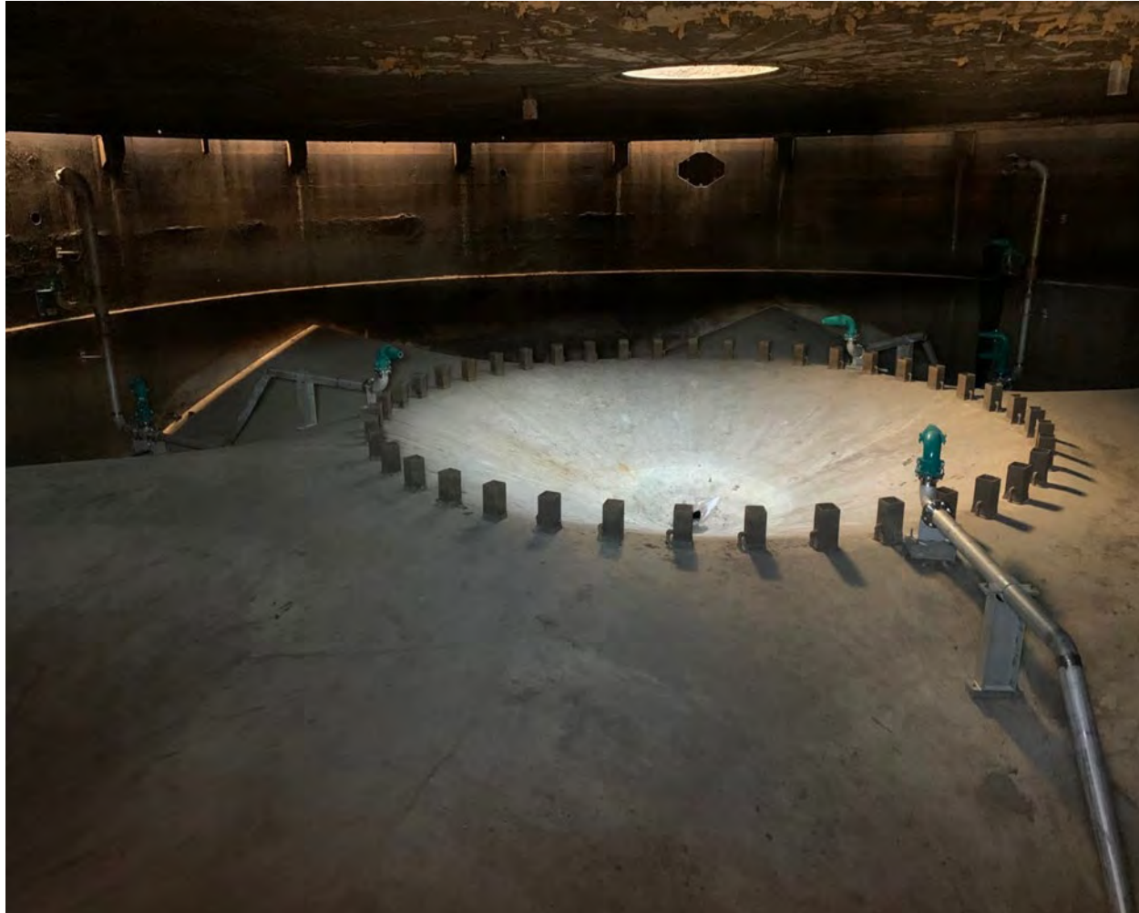
Pump Mixing System inside digester 1
